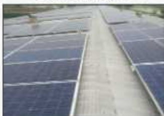
Industrial Shed-100KW Karnal, Haryana
