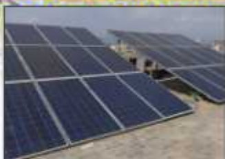
School Rooftop-10KW Dev Samaj School, Chandigarh
