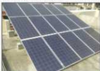
Factory Rooftop-25KW Sector 82 JLPL, Mohali
