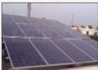
Residential Rooftop-10KW Zirakpur, Punjab
